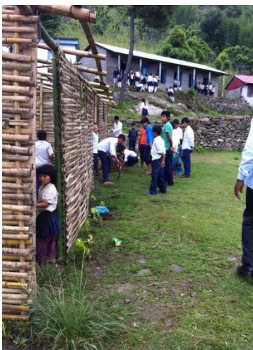
After the earthquake, temporary classrooms built from bamboo at the school in Deusa
