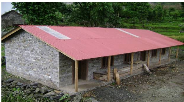
RRN propose building a one-storey two classroom block similar in design to the one under construction here (photo: RRN).
